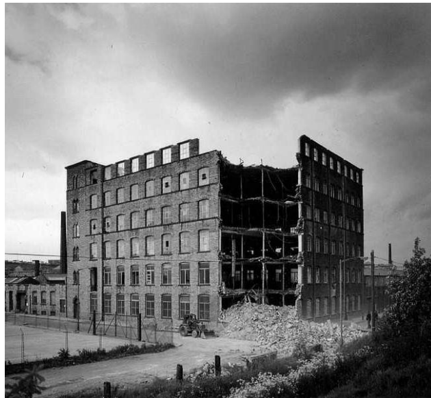
Figure 13. Mill under demolition in 1969 in Huddersfield, Yorkshire, England showing 'fireproof' iron frame with masonry jack-arch construction. Photo © by author.
