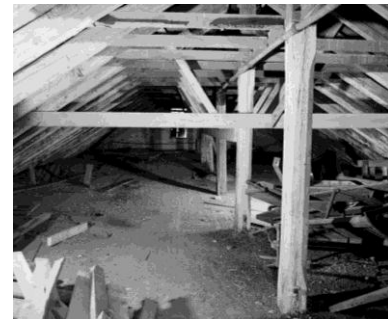
Figure 11. Interior of attic story showing characteristic fire-prone light frame gable roof construction.
