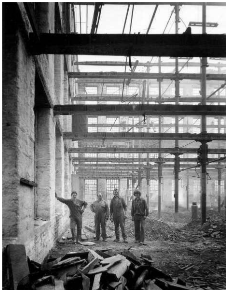
Figure 12. Mill under demolition in 1969 in West Riding area of Yorkshire, England showing iron frame with joist pockets visible on beams for wooden joists. Photo © by author.
