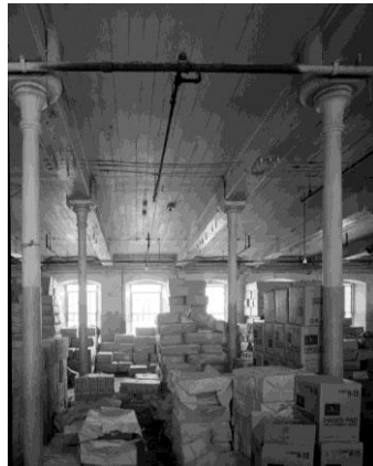
Figure 15. Interior of Stark Mill #2, Amoskeag Millyard, Manchester, N.H. showing beam-and-plank “ slow-burning ” construction, ca. 1840, before the term “ slow-burning ” was coined. This view shows an example of this system with a finished wood board ceiling nailed directly to the planks, with the 1” thick boards nailed crossways to the planks, parallel to the beams. Photo by the author for HABS.
