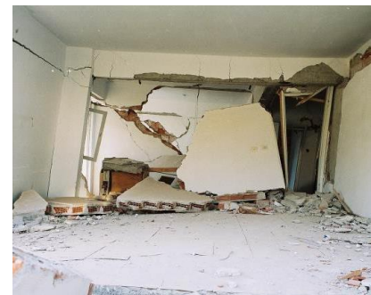
Figure 33: Collapsed RC building in 1999 showing shear failure of hollow clay tile infill wall.
