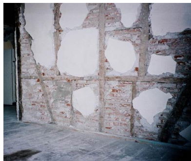
Figure 32: House in Düzce, Turkey after 1999 EQ, showing the ‘working’ of himis wall
