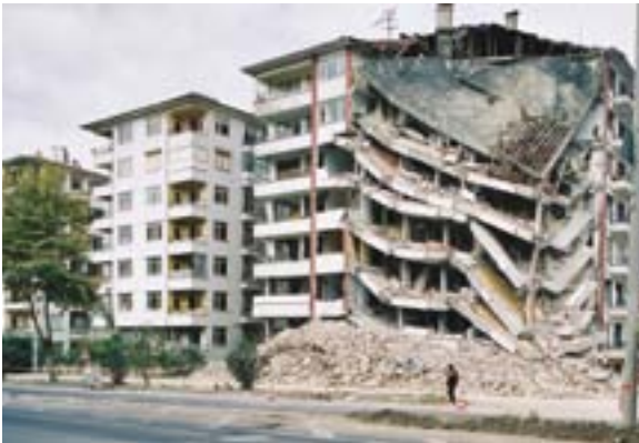
A multi-storey RC frame apartment house in Golcuk, Turkey partially collapsed by the 1999 earthquake. The lack of adequate moment connections and very thin columns is evident. © Randolph Langenbach
