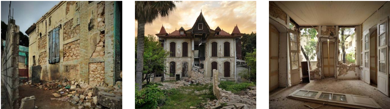
Figure 6. Brick and empanelled round-rock rubble stone construction, as is typically found in many of the Port-au-Prince “Gingerbread” Houses from the late 19th century, showing different levels of damage from onset, to collapse of the rubble panels. Center: The 2 ½ story Villa Castel Fleuri Mansion was of rubble stone between brick piers and window surrounds, and only the staircase projection collapsed. The onset of inelastic deformation of the rubble stone panels is visible where the surface stucco has come off. Right: The Dufort House still standing on its brick piers after the collapse of the rubble stone panels. This house is now being restored by FOKAL. Many reinforced concrete buildings nearby collapsed.
