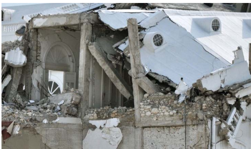
12. Detail view showing the reinforced concrete frame with round rock rubble stone infill of the 1916 structure exposed during the demolition of the ruins of the National Palace.
