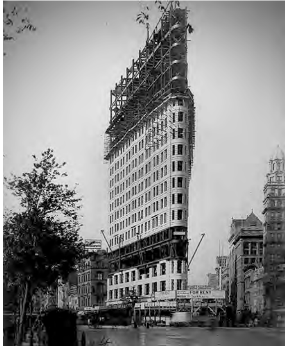
Fig. 3.12 Flatiron Building in New York City under construction in 1902 showing the heavy stone masonry façade resting on the steel frame. The upper walls were constructed separately probably to ensure the weight is bearing on the frame rather than the lower masonry walls. U.S. Library of Congress Photograph
