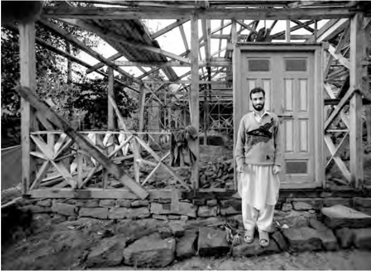
Fig. 3.19 The owner standing in front of his house under construction showing the light timber frame of dhajji construction before the rubble stone masonry with mud mortar infilling. His unreinforced rubble stone house had collapsed in the earthquake and he and his neighbors proceeded to rebuild with dhajji when they saw that the only house to survive in the village was the only one of dhajji construction and that the one building of RC construction had also collapsed. Photograph by © Randolph Langenbach
