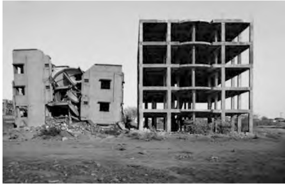
Fig. 3.16 Two RC frame buildings in Bhuj, India after the 2001 Gujarat earthquake. The building on the left had been completed, while the frame only of an identical building had been completed on the right. The earthquake collapsed the one where the frame was restrained by the masonry infill walls, while the bare frame survived. Photograph by © Randolph Langenbach
