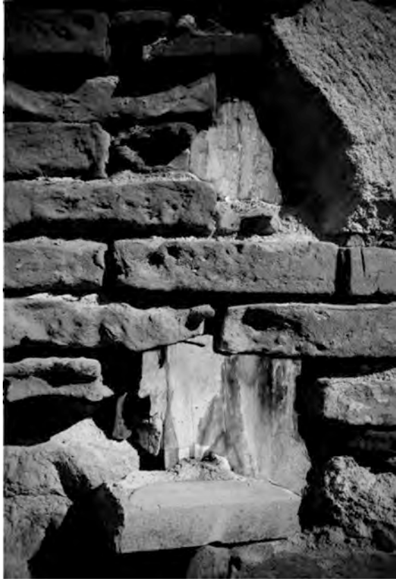
Fig. 3.8 A vertical column of the timber frame in the building in Fig. 3.7 showing through holes in the brickwork. Photograph by © Randolph Langenbach
