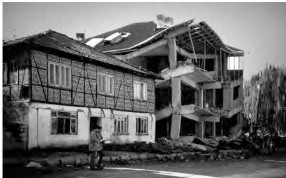
Fig. 3.17 A collapsed RC building next to a surviving hmuş building in Turkey after the 1999 earthquakes showing the resilience of the timber frame with masonry infill compared to that of a new RC frame building of modest height next door. It is interesting to compare this view with Fig. 3.16, where the infill probably caused the collapse, while here the infill and timber frame worked well together. Photograph courtesy of Adem Doğangün
