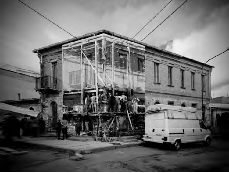
Fig. 3.7 An early 20th century building in Mileto, Calabria, Italy constructed with a baraccata timber frame embedded on the inside face of the wall, with a photo of it taken during its construction. Photo courtesy of the owner
