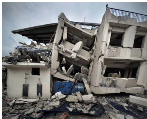
22. Reinforced concrete building in central Port-au-Prince nearly collapsed by the 2010 Haiti earthquake.
