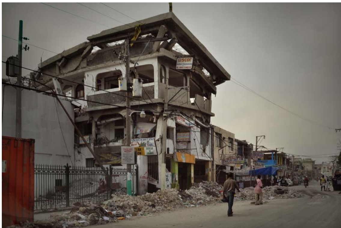
11. A downtown commercial building in a near state of collapse – illustrating the brittle vulnerable nature of many of the formal, contractor-built reinforced concrete buildings in Port-au-Prince. Many buildings of this type did pancake collapse, but, as demonstrated by the buildings on either side that are still intact, everything did not fall down. Approximately 40% of the buildings in the central city were partially or totally collapsed, but of the remaining 60%, many suffered little damage. ©Randolph Langenbach
