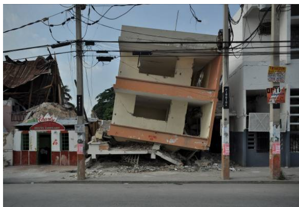
23. A formerly four story building in Port-au-Prince showing weak story collapse.
