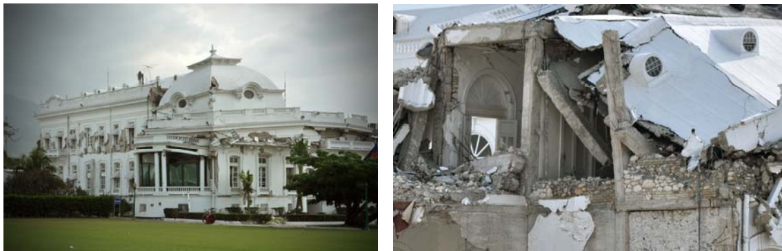
14. left : National Palace in Port-au-Prince after the earthquake and partial demolition, revealing the reinforced concrete frame infilled with rubble stone. The steel reinforcing bars in the exterior portions of the frame and poured concrete walls (visible on left side of left photo) were heavily corroded in this over 90 year old structure. Left : © Randolph Langenbach.
