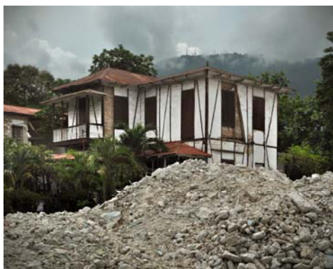
27. A Port-au-Prince house of colombage construction showing slight earthquake damage behind the rubble pile of a collapsed reinforced concrete building.
