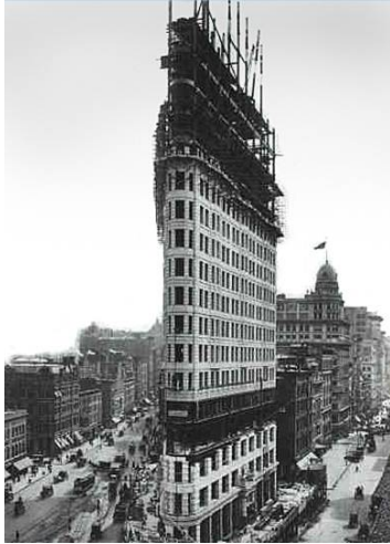
17. Flatiron Building in New York City under construction in 1902 showing the heavy stone masonry façade resting on the steel frame. The upper walls are constructed separately probably to ensure the weight is bearing on the frame rather than the lower masonry walls.
