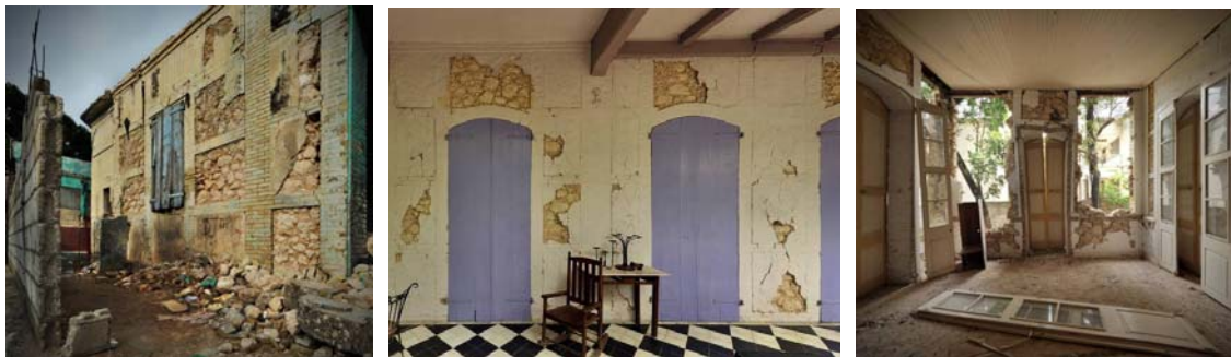
10. Brick and empanelled rubble stone construction, as is typically found in many of the Port-au-Prince "Gingerbread" Houses from the late 19 th century, showing different levels of damage from onset, to collapse of the rubble panels. Surprisingly few houses with this construction collapsed overall, despite the weakness and vulnerability to earthquake shaking of this construction – a further verification that the intensity did not exceed MMI-VII at these Port-au-Prince sites. © Randolph Langenbach
