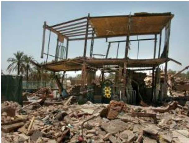
Fig. 3. Light steel frame building with jack-arch floors and roof damaged in the 2003 Bam earthquake.
