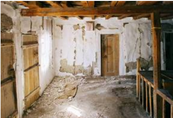
Fig. 26. Interior of a traditional house in Yuva, Turkey of after the 2000 Orta earthquake showing evidence of the working of the hımış walls.
