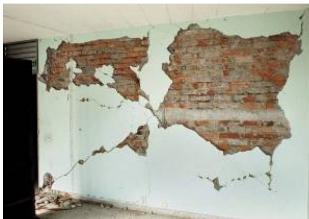
Fig. 29. Typical infill masonry wall found inside the upper stories of the building in Fig. 28 showing that the infill wall was subdivided with a concrete beam and column similar to that advocated for Armature Crosswalls.
