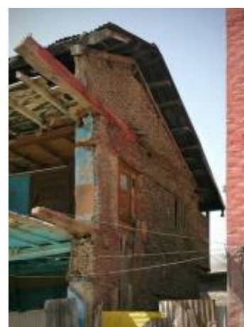
Fig. 11. A partially demolished building showing timber-laced masonry bearing wall typical of taq construction.
