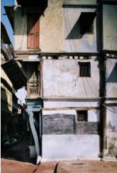
Fig. 14. Timber-laced four story masonry building in historic center of Ahmedabad after 2001 earthquake.
