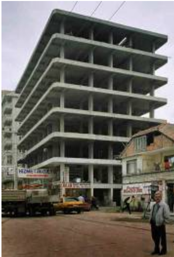
Fig. 24. Building under construction in Gölcük, Turkey shown after the 1999 earthquake. Because the masonry infill walls had not yet been installed, frame action was able to occur, and thus the building was not collapsed by the earthquake.
