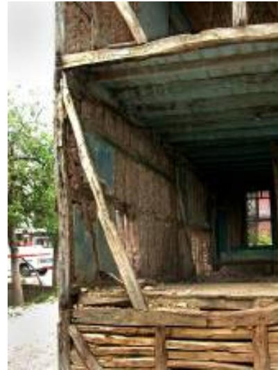
Fig. 6. The interior face of the same wall in Fig. 5. Despite its condition, the 1999 Kocaeli earthquake which caused the collapse of hundreds of nearby modern buildings, had little effect on it.
