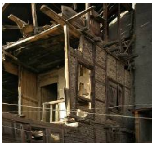
Fig. 10. A partially demolished dhajji dewari building showing timber frame with infill masonry construction.
