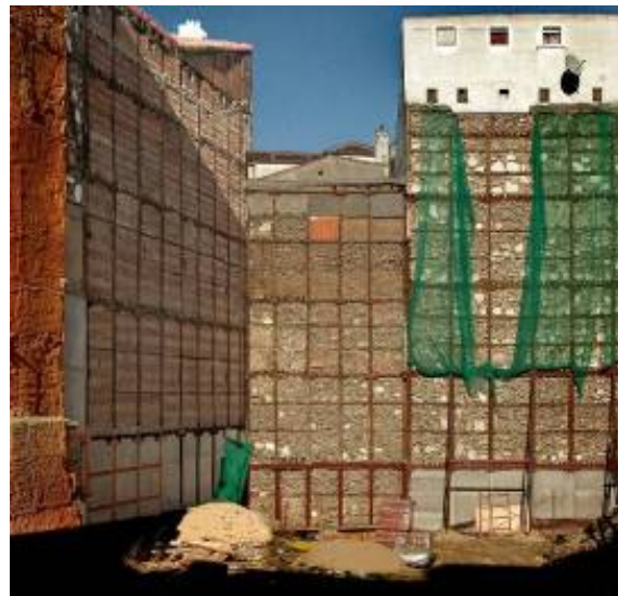
Fig. 13. Backs of 5 to 7 story buildings in central Madrid exposed by demolition of adjacent structures showing the timber frame construction with rubble masonry infill typical of the area in the 17 th -19 th centuries.
