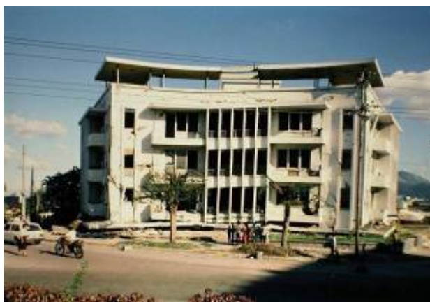
Fig.28. Apartment block in San Salvador that suffered a soft-story collapse in the 1986 San Salvador earthquake. The progressive collapse of the upper floors was stopped by the resistance of the infill masonry.
