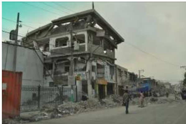
Fig. 19. Reinforced concrete building in central Port-au-Prince nearly collapsed by the 2010 Haiti earthquake.
