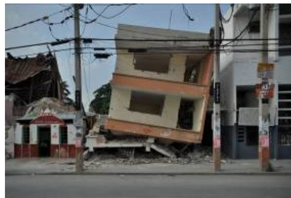
Fig. 20. A formerly four story building in Port-au-Prince showing weak story collapse.
