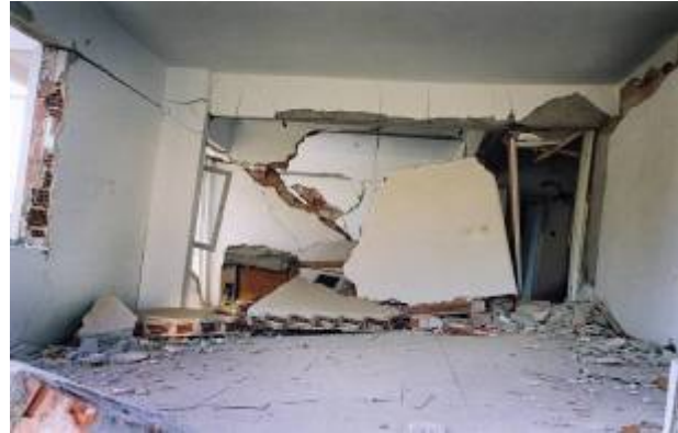
Fig. 27. Typical hollow clay tile masonry wall in a reinforced concrete apartment building in Gölcük, Turkey collapsed by the 1999 Kocaeli earthquake.
