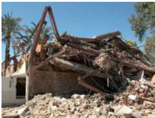
Fig. 7. Steel frame building collapsed by the 2003 Bam, Iran earthquake.
