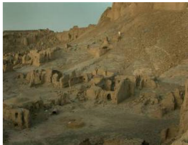
Fig. 31. The unrestored ruins in the Konari neighborhood of the Arg -e-Bam after the earthquake. Although abandoned and untouched for more than 150 years, these structures survived the earthquake with comparatively little damage.
