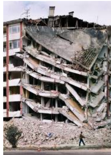
Fig. 25. Building in Gölcük close to the one shown in Fig. 17 collapsed by 1999 earthquake. The heavy masonry infill walls together with open (soft) ground floors were often contributors to such collapses.
