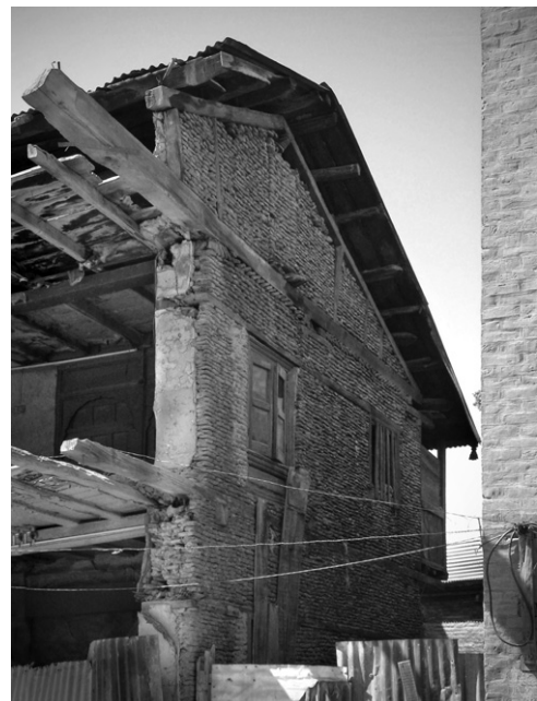
Fig. 3. Partially demolished taq construction (Srinagar, Kashmir, 2006) showing timber lacing laid into the wall. Timber bands at floor level and at the window lintel levels.
