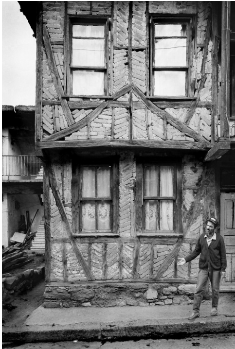
Fig. 1. This long abandoned and unmaintained 2.5 story humuş house in Gölcük survived the 1999 earthquake with little additional damage, despite the widespread collapse of the surrounding RC structures.
