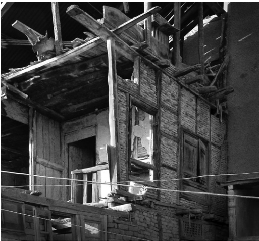
Fig. 4. Partially demolished dhajji dewari construction Srinagar, 2007). Timbers form a complete frame with only a thin single layer of masonry infill; interlocking of timber joists with the exterior wall is visible — a key seismic feature to taq and dhajji dewari .
