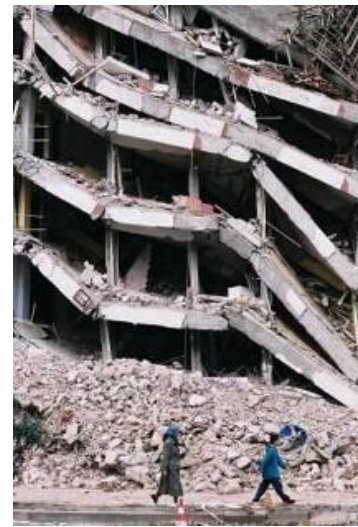
Figure 19: Partial collapse of RC Building, Gölcük , Turkey, 1999.
