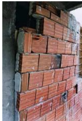
Figure 24: Infill wall RC building in Mexico City damaged in 1985 earthquake. The infill masonry in this structure almost caused the collapse of the building. The damage to the corner column that left the building teetering on the edge of collapse can be seen on the right.
