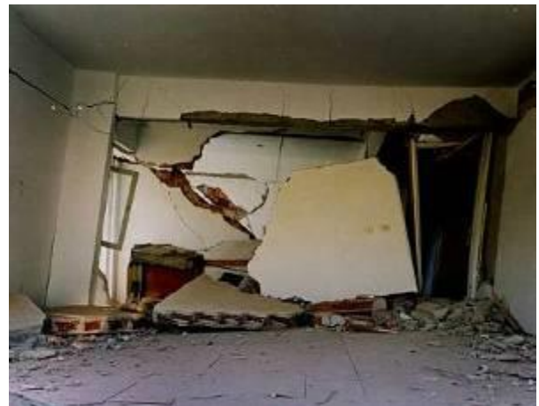
Figure 31: Collapse of a brittle interior hollow clay block wall illustrating typical failure pattern for such walls lacking subdivisions.
