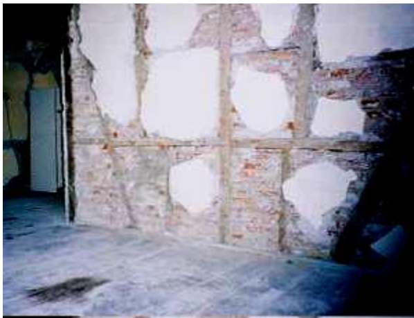
Figure 30: Hımış interior wall in house in Düzce earthquake damage district showing “working” of wall that caused loss of plaster.
