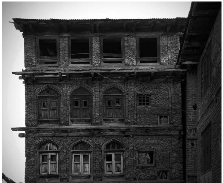
Fig. 6 Example of taq construction in Srinagar, Kashmir, 2005. The timbers in the masonry walls only run horizontally parallel to the wall and through the wall (photograph © Randolph Langenbach)
