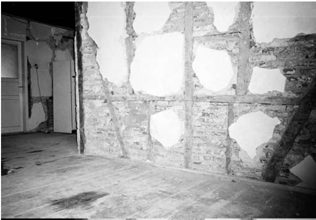
Fig. 12 Hımış interior wall in a house in the Düzce earthquake damage district showing »working« of wall that caused loss of plaster (photograph © Randolph Langenbach)
