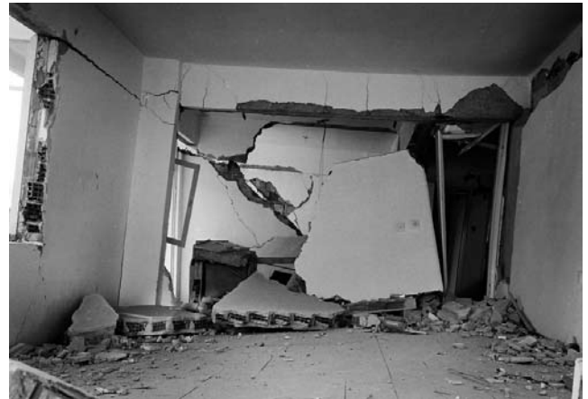
Fig. 13 Collapse of a brittle interior hollow clay block wall illustrating typical failure pattern for such walls lacking subdivision of the masonry (photograph © Randolph Langenbach)
