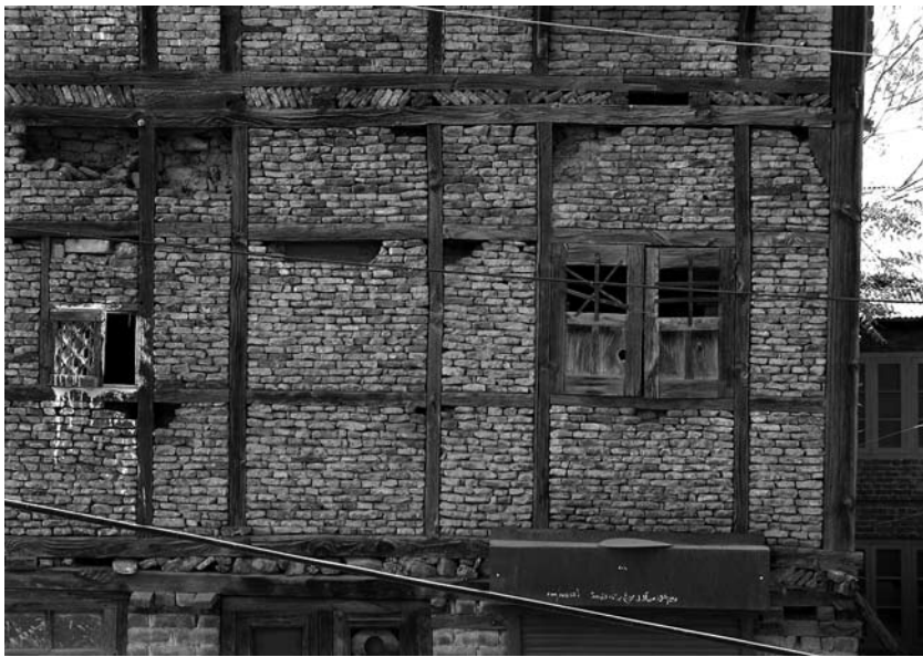
Fig. 7 Example of dhajji dewari construction in Srinagar, 2005. The timbers form a complete frame, and the masonry is inset into the frame (photograph © Randolph Langenbach)
