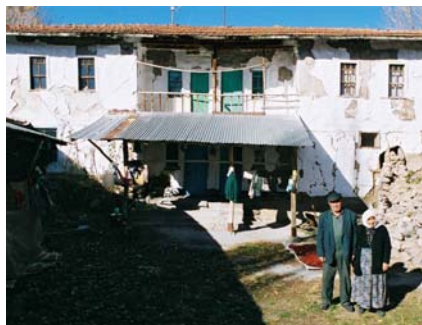
Traditional house in Yuva with repairable damage that was condemned by government engineers after the 2000 Orta earthquake.
