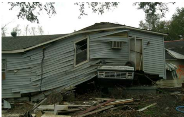
Damage from levee break in Lower 9 th Ward, New Orleans after Hurricane Katrina.
