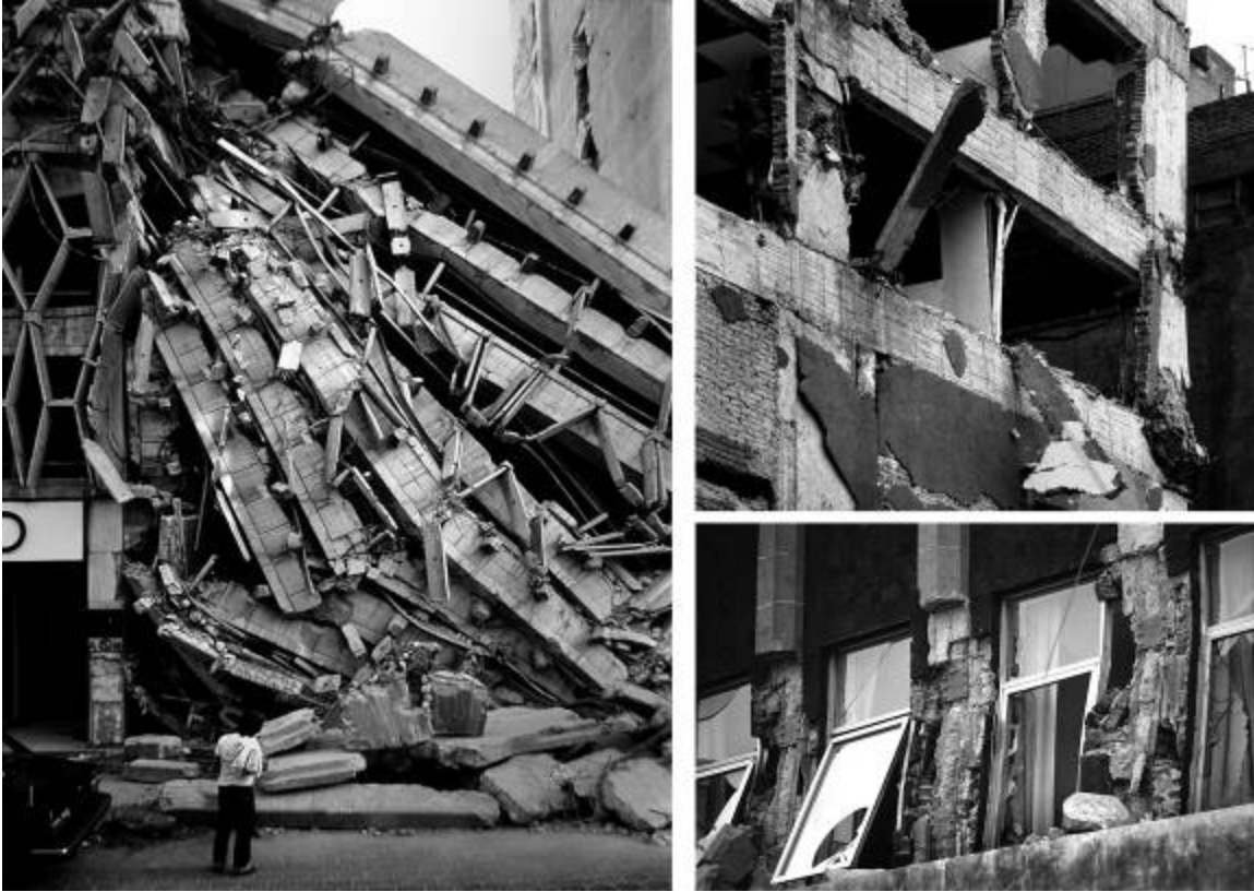
Figure 11. Mexico City 1985 earthquake: (L) Collapsed RC Parking garage. (C) RC frame showing column damage and loss of infill. (R) Bent steel frame in ca.1940 building with too little masonry to help.
