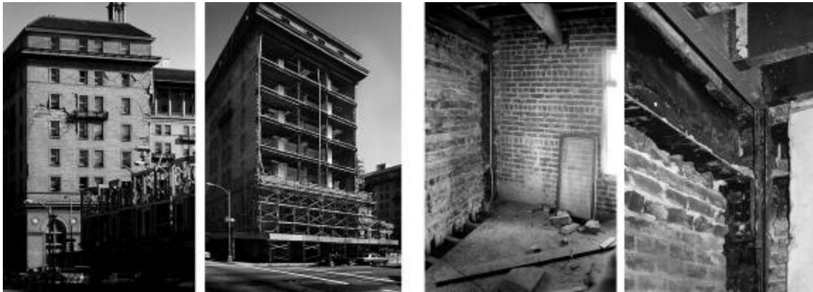
Figure 9. (L) The Oakland Hotel showing damage to façade, and later during repairs. (R) The Touraine Hotel, Oakland, California showing masonry exterior infill during upgrade work.
