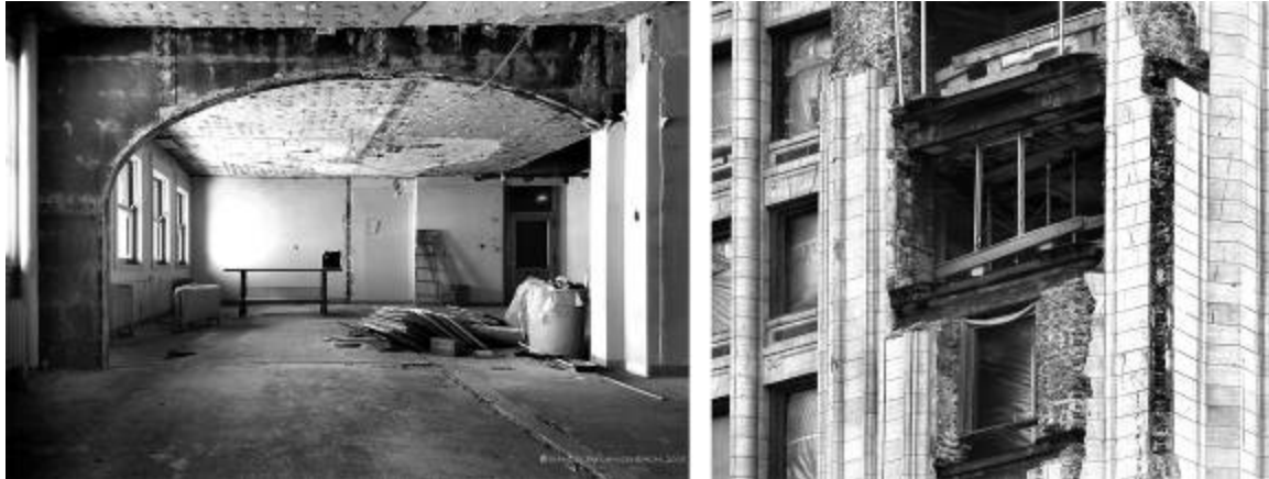
Figure 6. (L) Portal arch wind bracing in Monadnock Building, South Half (1891-3). (R) Cladding on 90 West Street (1907) damaged by World Trade Towers collapse showing steel shelf angles.
