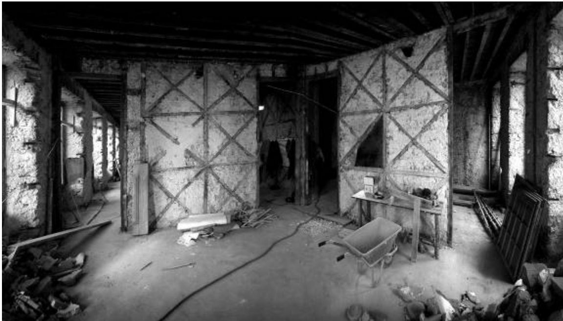
Figure 13. Interior of late 18 th Century building with Pombalino walls revealed during renovation work in 2003. This example does not have the gaiola frame extending into the exterior masonry.
