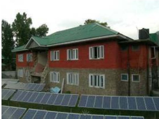
Figure 32: Adjacent annex to medical clinic was only slightly damaged except for the collapse of the walls of the stairway, which rendered it unusable.
