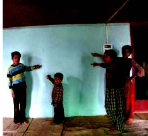
Figure 13: Interior of ca. 1900 house in Baramula showing cracks where the people are pointing. The cracks are limited to plaster cracks around the Dhajji Dewari infill panels.
