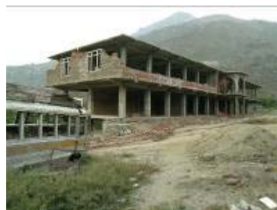
Figure 38: Reinforced Concrete structure under construction at time of earthquake. Undamaged, except for out-of-plane collapse of some infill masonry.
