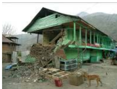
Figure 37: Rubble masonry building with all walls collapsed but front where balcony and timber door frames held the stone together.
