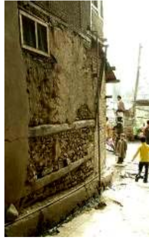
Figure 12: Timber lacing in URM wall of house in Baramula.
