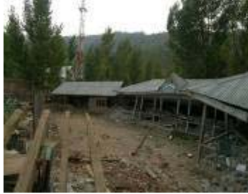
Figure 26: Collapsed School buildings in Uri Government Complex.
