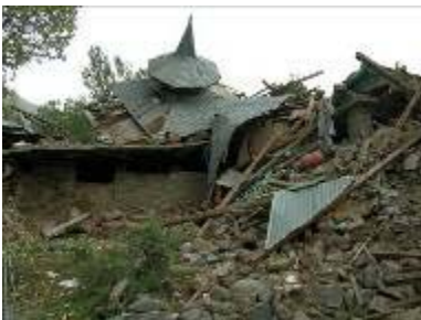
Figure 28: Collapsed Mosque in Uri Government complex.
