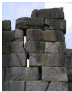
Figure 15. Top right corner of wall in Fig.14.
