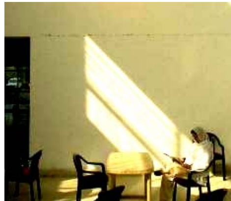
Figure 4: This crack shows how minor the earthquake damage is, because it is only the propagation through the surface plaster of the interface between infill and the RC frame.
