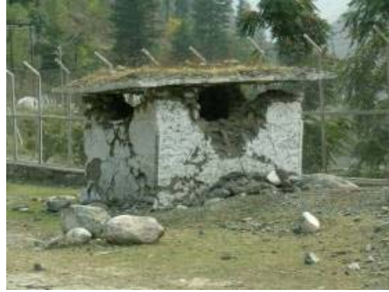
Figure 22: A small military structure near to the Detha Mandir Temple provides an example of damage associated with rigid concrete roofs on rubble masonry walls. A nearby similar structure with a timber and heavy sod roof remained completely intact.
