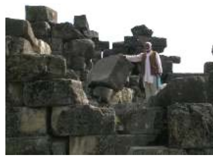
Figure 16: This large stone block under the man's hand is the only block to fall off the wall in the earthquake.
