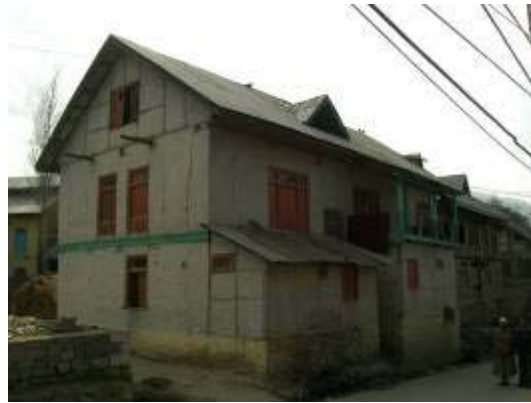
Figure 17: Taq construction house where movement from the earthquake reveals where the masonry panels are disconnected from the piers.
