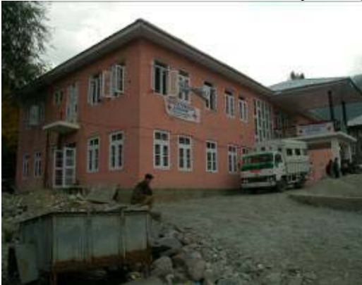
Figure 31: This Medical Clinic in Uri Government complex was not significantly damaged, and is still in use.
