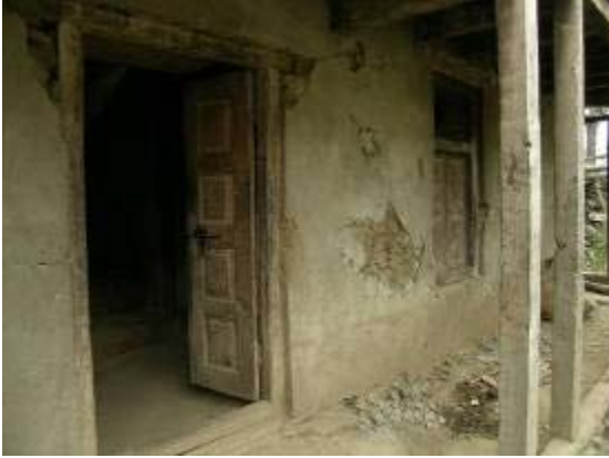
Figure 23: The earthquake caused stresses in the ground floor wall to cause the shedding of the concrete stucco, but the horizontal timber lacing helped hold the wall from cracking and collapsing.
