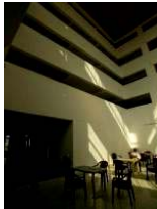
Figure 4: Interior of five story Heemal Hotel showing location of crack in figure 5.
