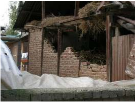
Figure 16: Dhajji Dewari wall in barn that partially collapsed because of insect infested timbers.
