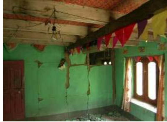
Figure 24: The interior of the same house shows how the plaster cracks reveal the location of the Dhajji Dewari construction infill panels.
