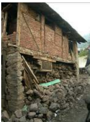
Figure 36: Intact Dhajji Dewari wall above collapsed rubble masonry wall.
