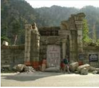
Figure 18: Buniyar Temple gate showing fallen stones from the collapsed column and top lintel.
