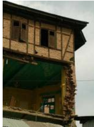
Figure 10: Detail of collapsed wall in building shown in Figure 9.
