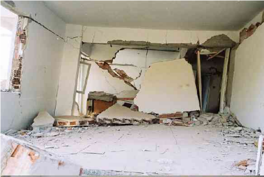
Figure 14: Collapsed interior infill wall in reinforced concrete building in Gölcük
