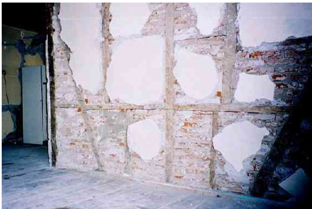
Figure 12: Hımış interior wall in Düzce after earthquake.
