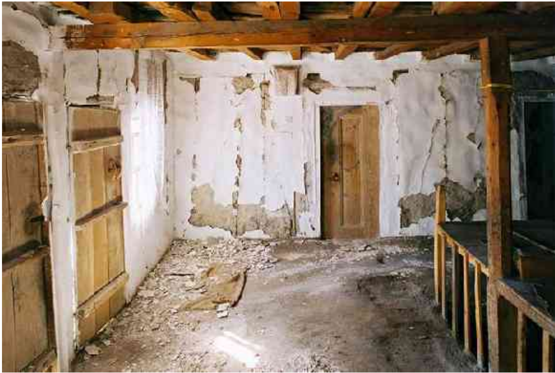
Figure 13: Interior of hımiş house in Orta after earthquake showing damage to mud and lime plaster over infill walls.
