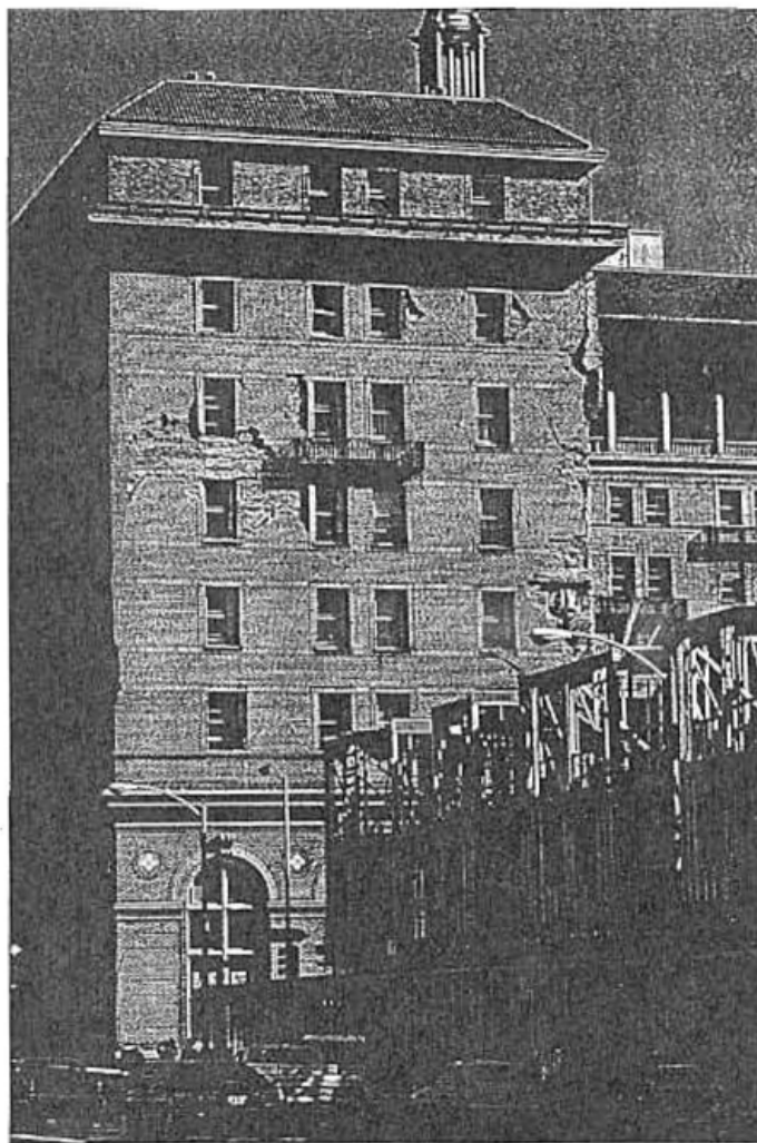
THE REMOVAL, PRIOR TO THE LOMA PRIETA QUAKE, OF INTERIOR MASONRY PARTITIONS FROM THE HOTEL OAKLAND MAY HAVE CONTRIBUTED TO THAT STRUCTURE'S DAMAGE. WITHOUT THE PARTITIONS, ALL OF THE LOADS HAD TO BE CARRIED BY THE REMAINING MASONRY OF THE EXTERIOR FACADE. PHOTO BY RANDOLPH LAGENBACH.
