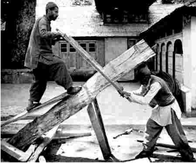
Pre-industrial building methods are still used in India. This ancient method of cutting timber into planks is not uncommon in this village in Kashmir.
