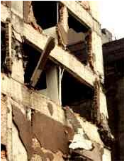
Victims of the 1985 Mexico City earthquake, the reinforced concrete columns on the right of this building have been damaged almost to the point of collapse by the "equivalent diagonal strut" effect of the infill masonry.
