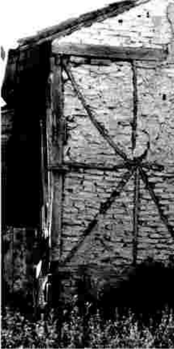
The brick-nogged construction shown here survived the great earthquake of 1963 in Skopje, Yugoslavia.
