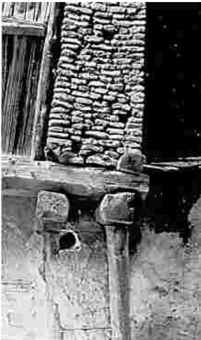
A typical masonry-wood connection in Kashmiri construction. These wood brackets are ubiquitous in both TAQ and DHAJJI-DEWARI structures. The masonry simply rests on top of the wood beams.
