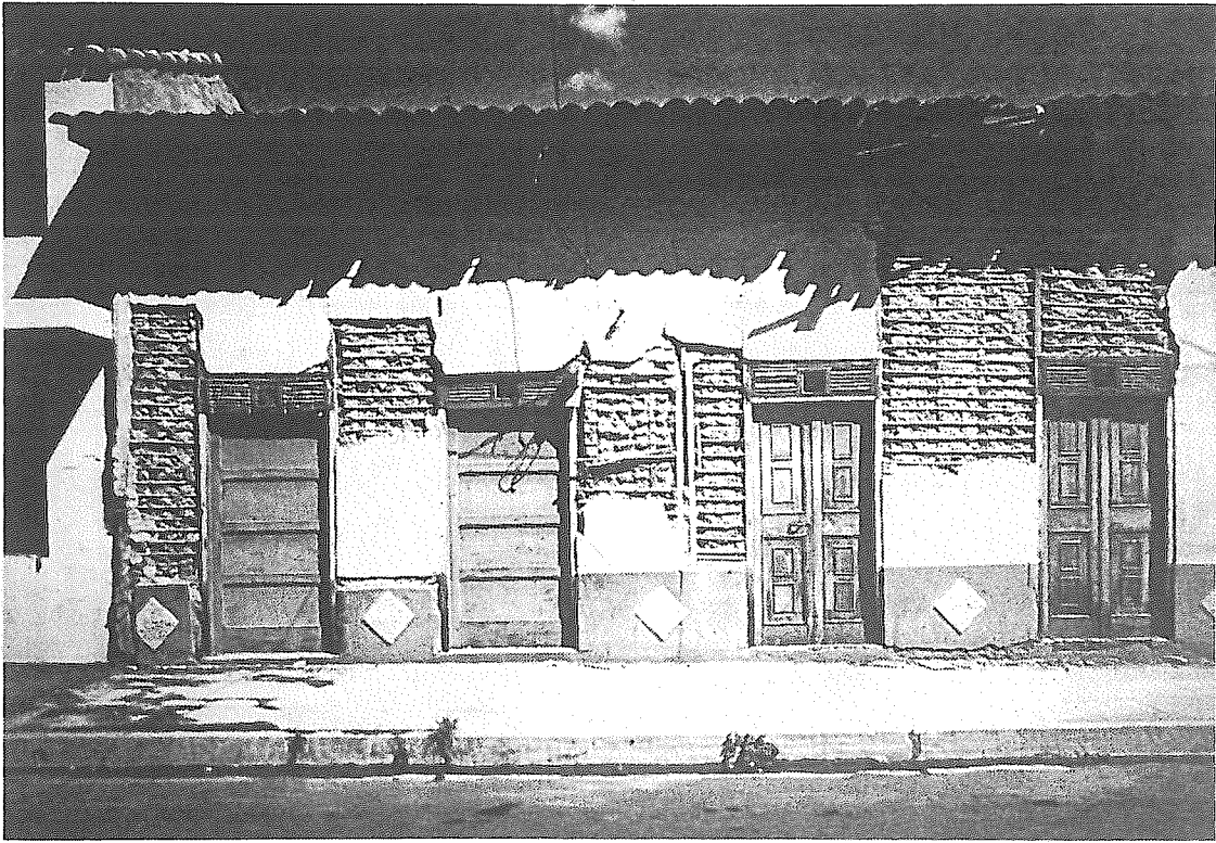
8. SAN SALVADOR, "Bahareque" building showing the shedding of stucco caused by the 1986 Earthquake.
