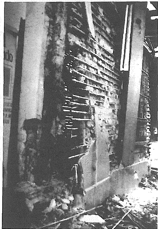
7. SAN SALVADOR, a "Bahareque" building damaged by the 1986 Earthquake showing how the failure began at the rotten base of the timber frame.
