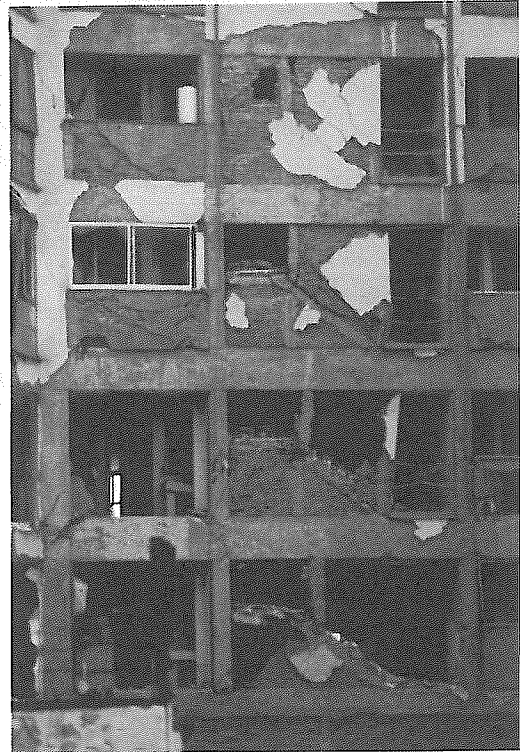
11. MEXICO CITY, reinforced concrete frame building showing the blowing out of the unreinforced brick infill walls and damage to the structural frame.
