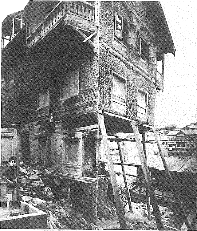
4. SRINAGAR, KASHMIR, INDIA, "Dhaji-Dwari" building undergoing repair demonstrating the through-wall bearing of the masonry onto the wood runners, and the comparative lightness of the masonry walls.
