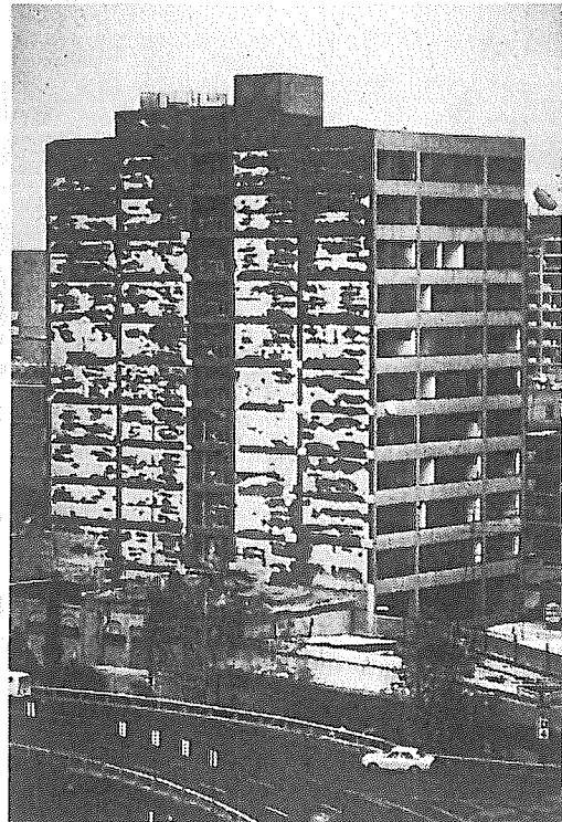
13. MEXICO CITY, eleven story building showing the absorption of shear stresses in the infill walls with the resulting shedding of the stucco.
